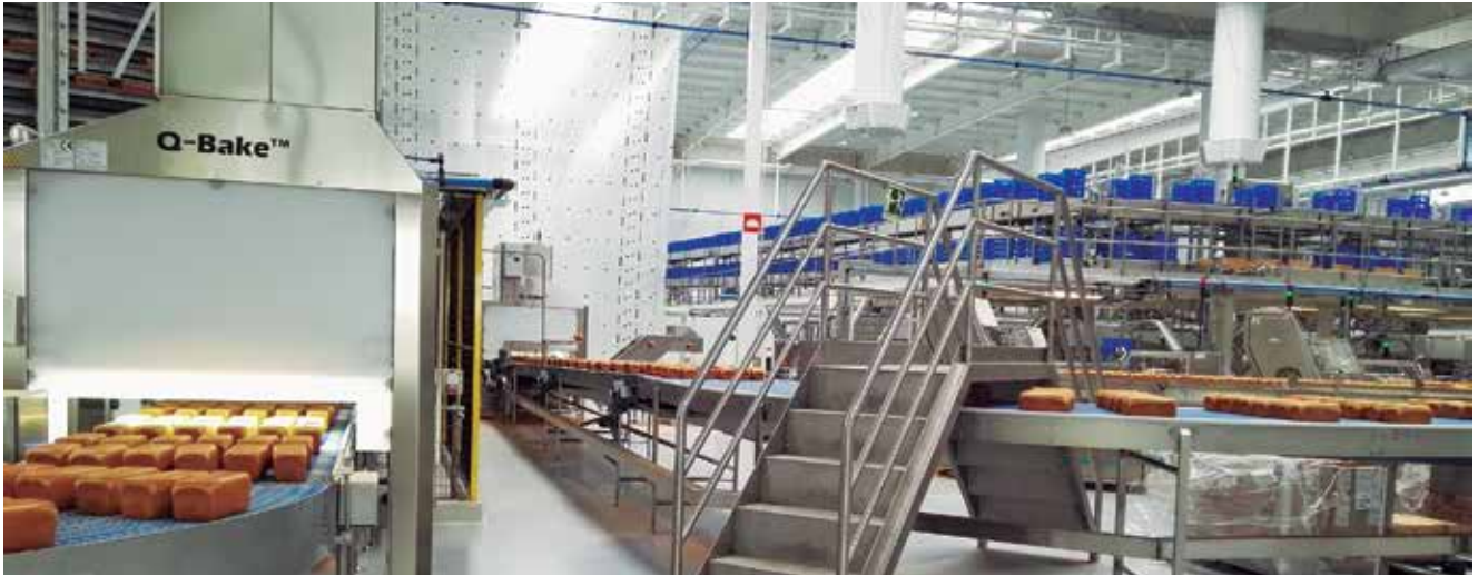
Mechanical works and conditioning system of the factory of Grupo Bimbo in Azuqueca de Henares, Guadalajara.
